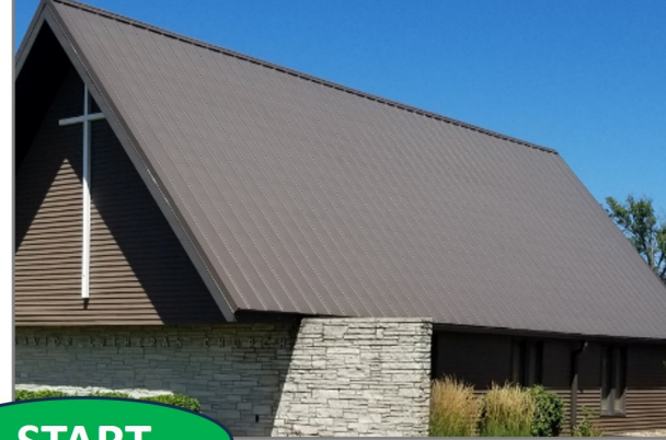
Hail Damaged Steel Roof
